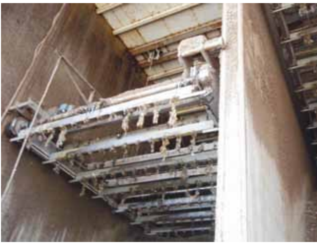
Figure 6. RDF storage system. Manufacturer: Vecoplan. (Source: MVW Lechtenberg).
